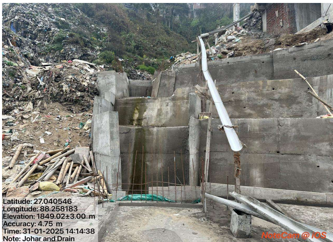
JHORA (DROP GUIDE) AND STORM WATER
